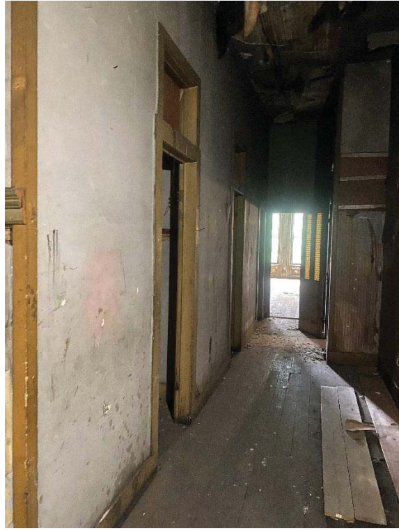
Image taken from the southern end of the second floor facing north, showing original entrances to former apartment units
