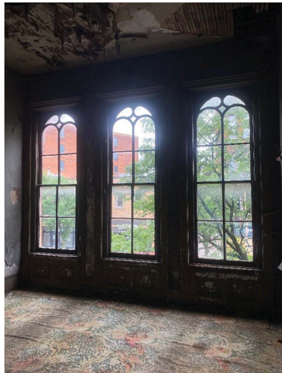
Image of the windows with a north view on the second floor of the property
