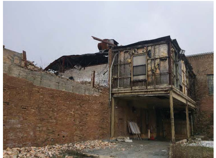
View southeast from the north side of the mill to fire damaged section of the mill.
