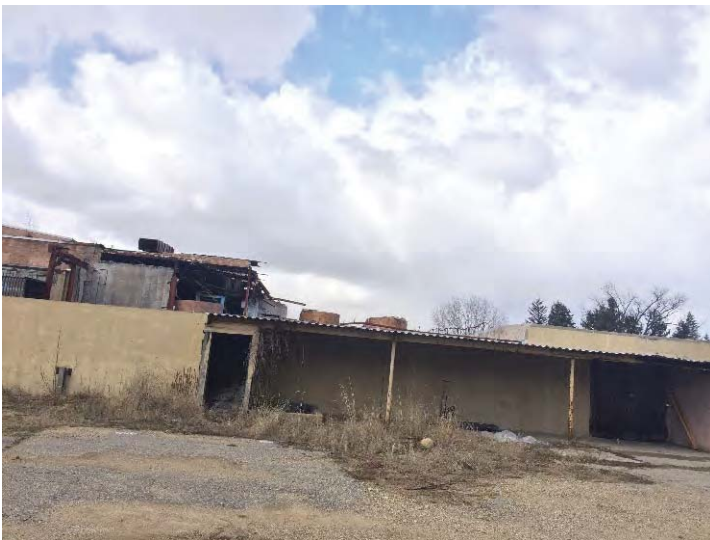
View west on the north end of the east side of the mill. Fire damaged buildings are in the background.
