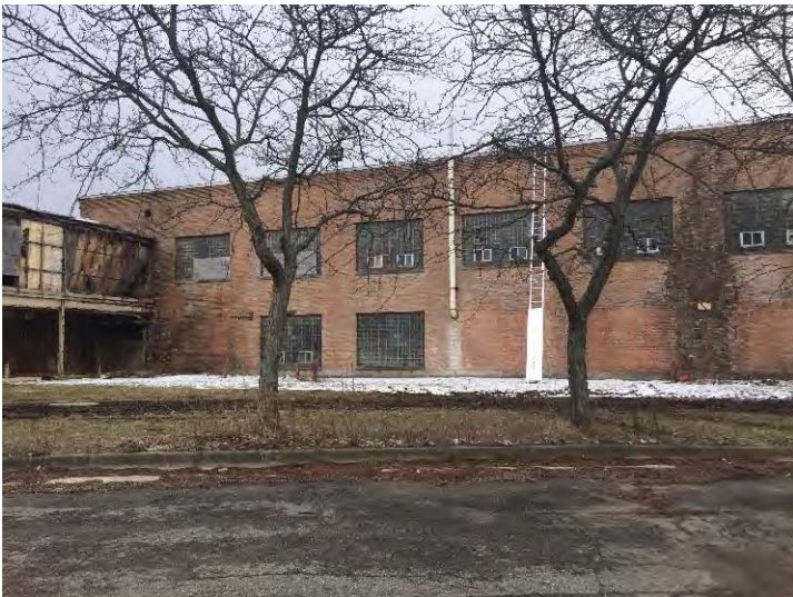
View southeast to the eastern portion of the north side of the mill. Fire damaged sections are present to the left.
