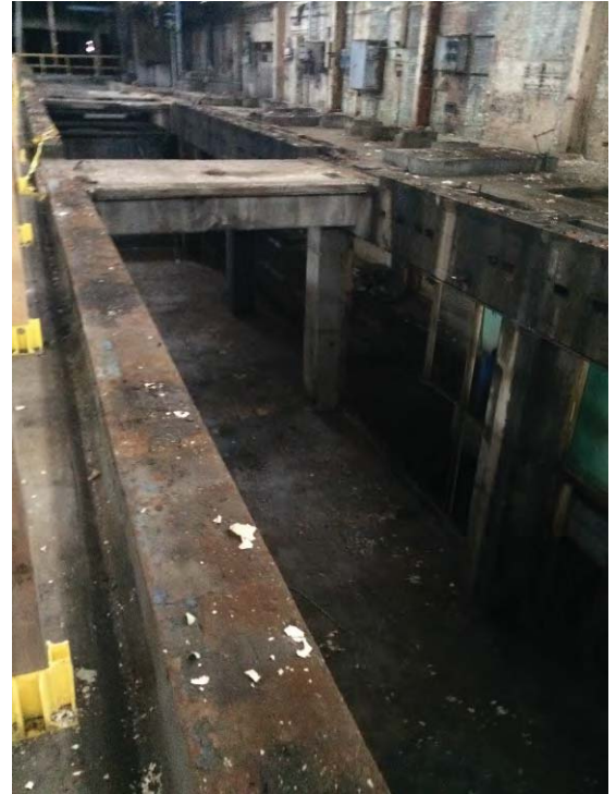
View to lower level in machine room.
