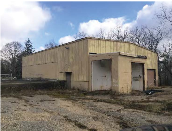
View northeast to the wastewater process building. On the right is the vault filled with water.
