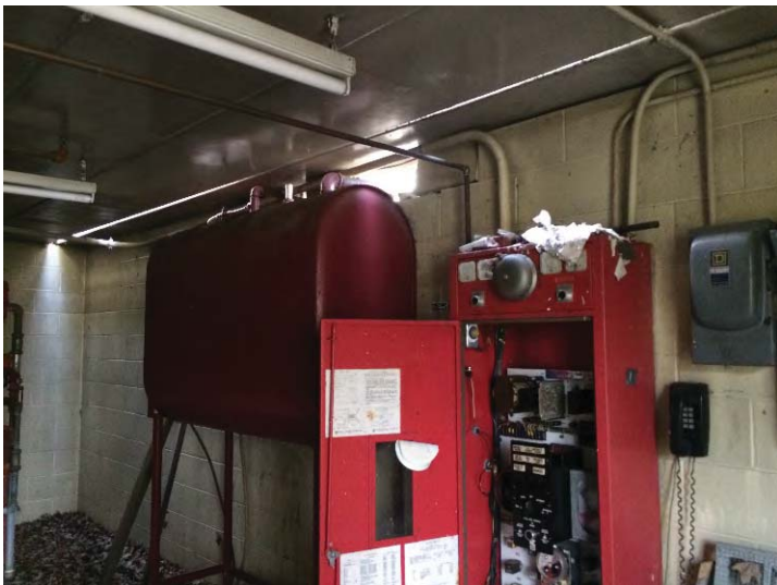
Interior of fire suppression building.
