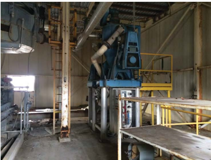
Interior of sludge handling building.
