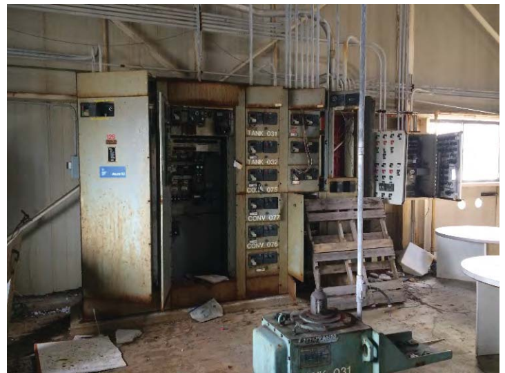
Interior of sludge handling building.
