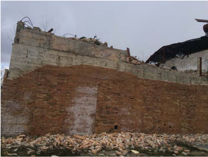
View east from the north side of the mill to fire damaged section of the mill.
