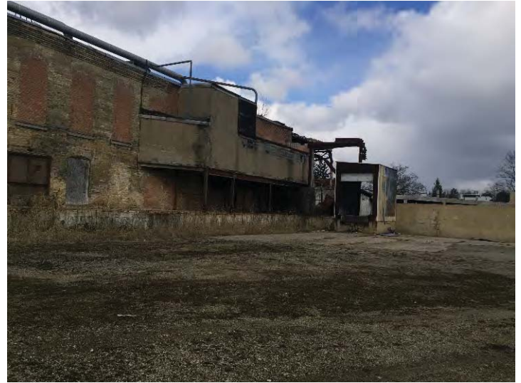
View northwest to the north end of the east side of the mill.
