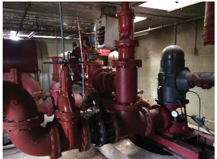
Interior of fire suppression building.
