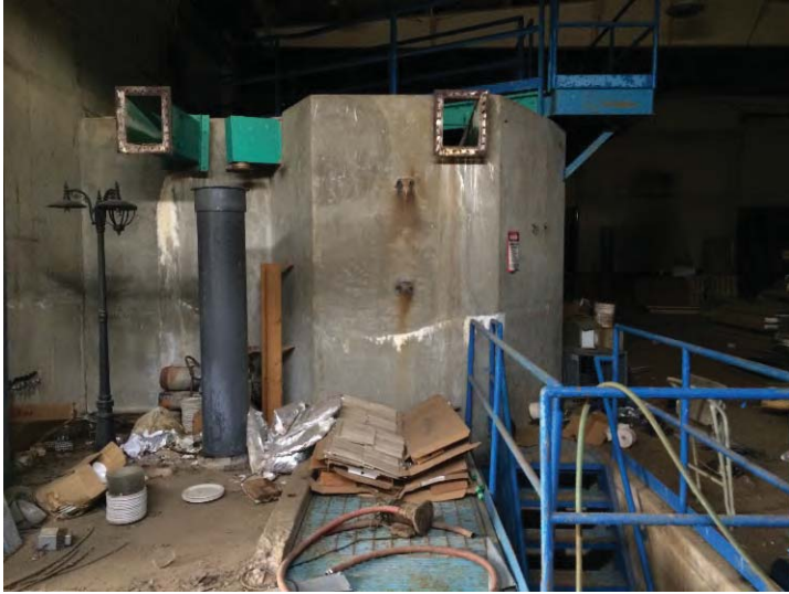
Interior of wastewater process building. Storage tank in the center.
