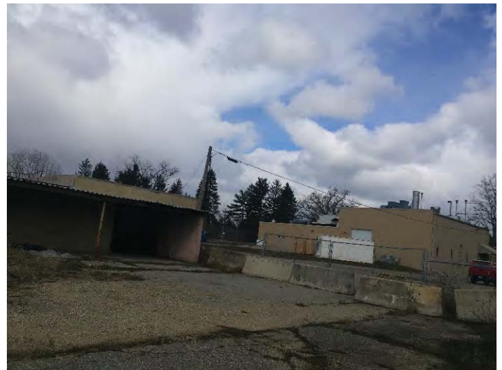
View to the north end of the east side of the mill with Bridge Organics, and adjoining property, in the background.
